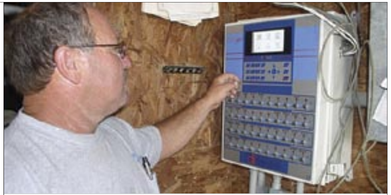
A computerized controller is programmed to manage the environment in a upgraded poultry houses.
